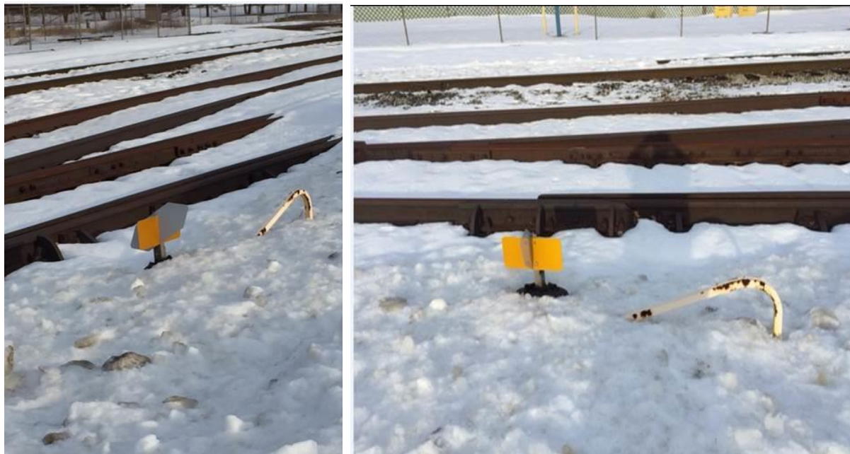
Improperly cleaned out switch:
