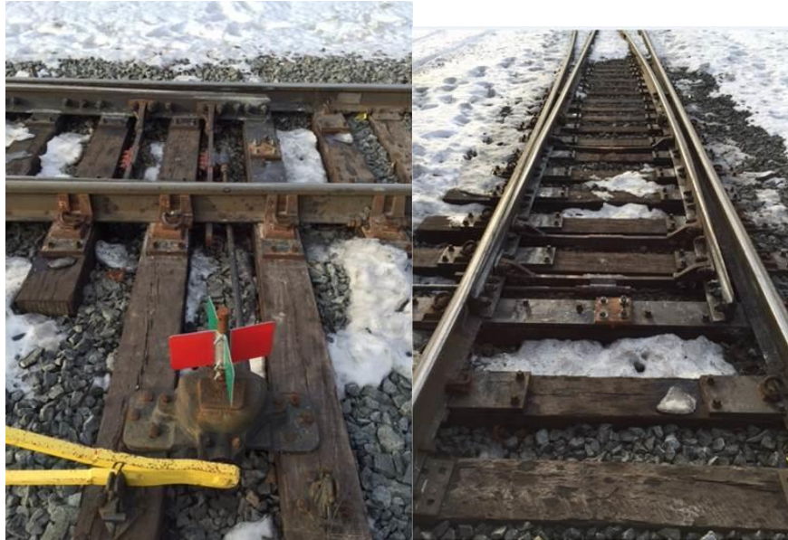
Properly Cleaned out switch:
