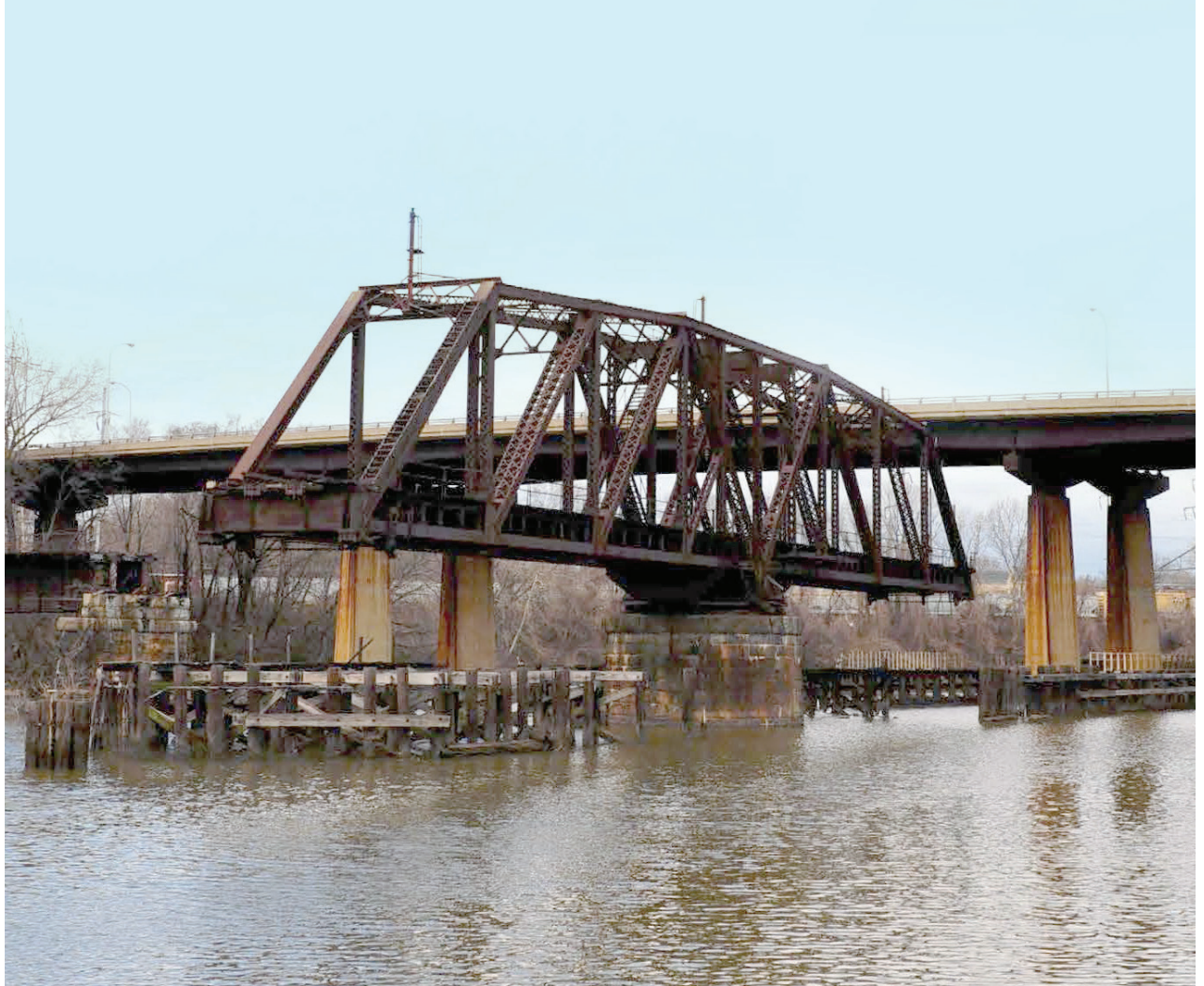
2014 view of the PW&B Swing Bridge (Bridge No. 31) in the open position, prior to its demolition. The 1976 Gray's Ferry Avenue Highway Bridge is in the background.
